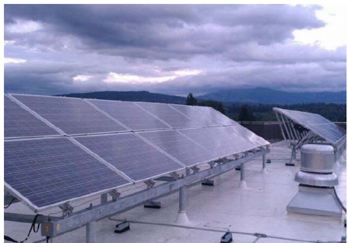
Solar array on the roof of Lincoln Square
