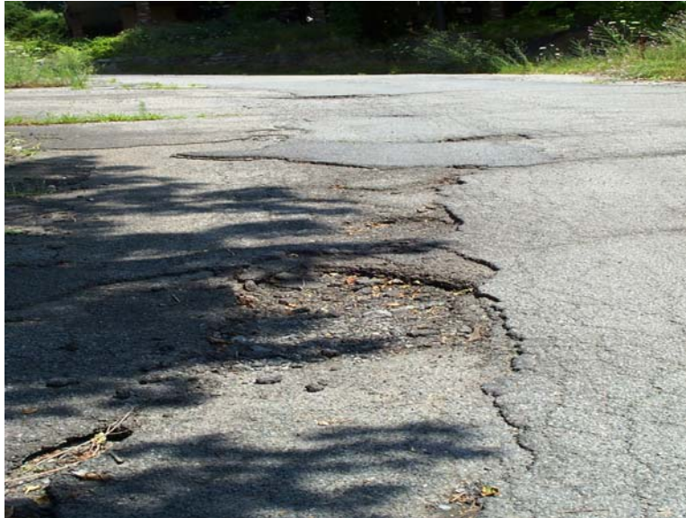
Pavement deterioration in the parking facility
