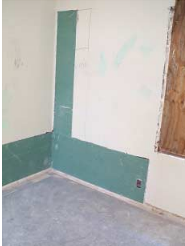
Photo of Potrero Annex building with modernization in-progress. Photo showed only section of interior drywall removed and replaced.
