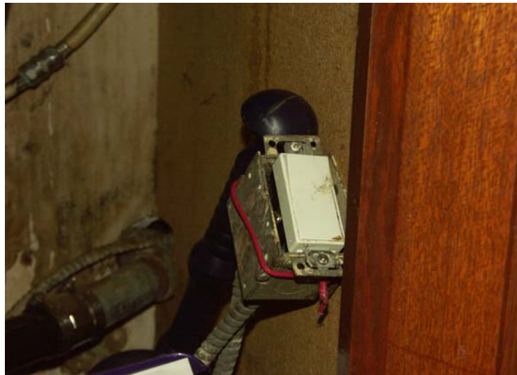
Exposed electrical wiring on/off switch for garbage disposal
