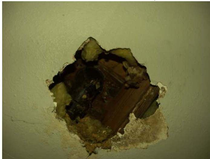
Hole in the ceiling.
