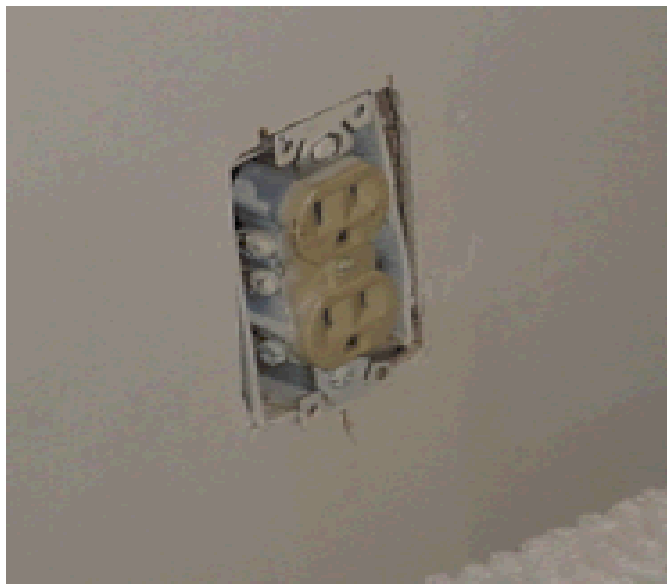
Missing outlet cover, creating an electrical shock hazard.
