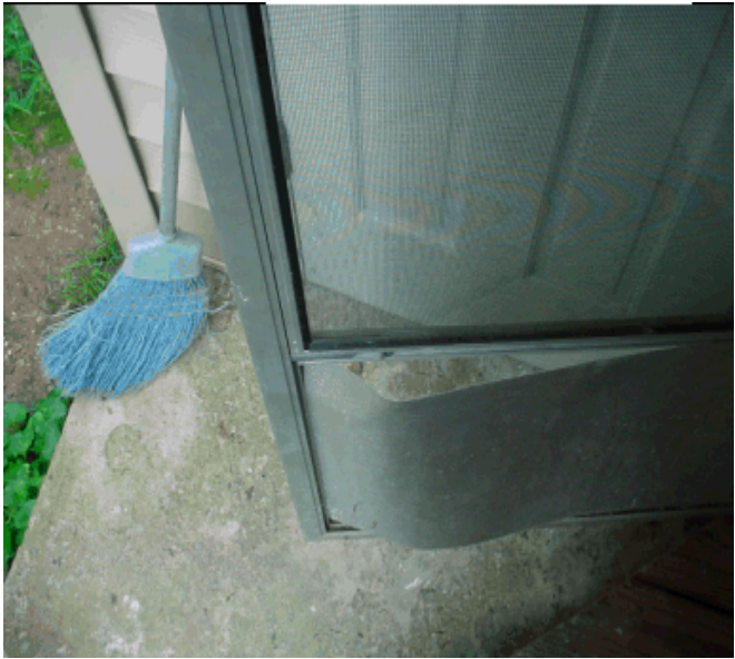
Cutting hazard on screen door that Authority did not report during June 24, 2005, inspection.
