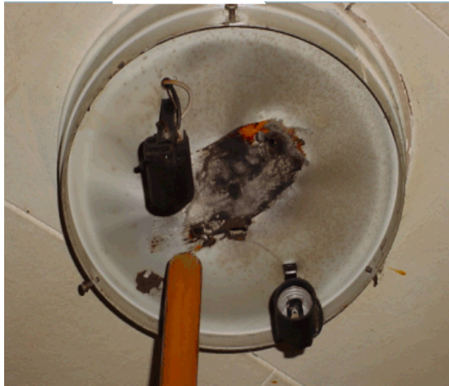
Burned kitchen light fixture with exposed wiring. Tenant stated that this deficiency had existed for more than two years.
