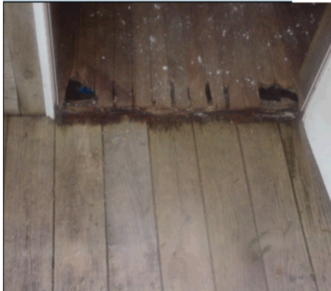
Holes and rotting wood in floor where kitchen meets back porch.
