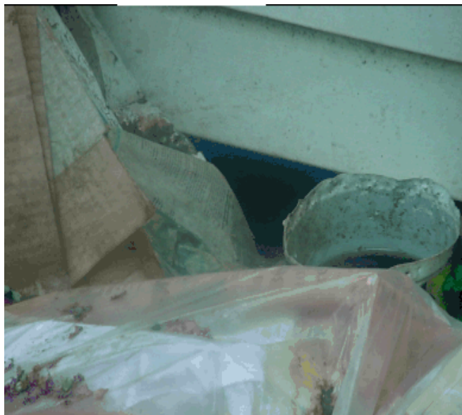
Hole in foundation that Authority did not report as a deficiency during its May 10, 2005, inspection.
