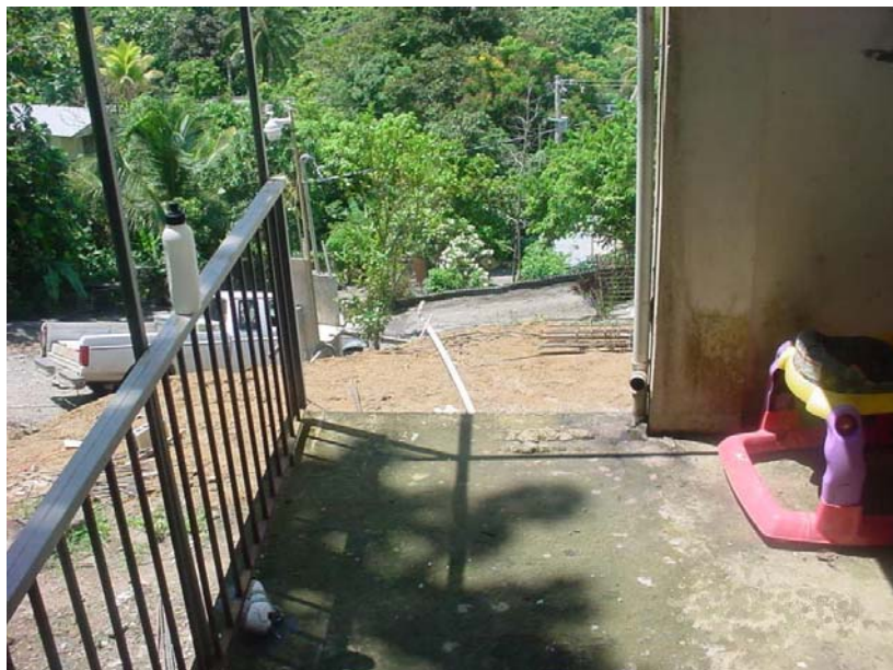
Second floor porch with missing handrails. The tenant stated that this deficiency had existed since move-in, around September 2004.
