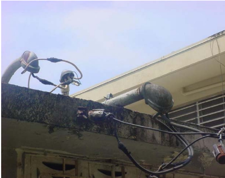
Main electrical connection hanging from pole within reach, creating an electrical shock hazard. The deficiency was not reported by the Authority during its July 12, 2005 inspection.
