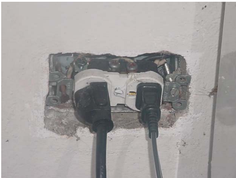
Missing outlet cover, creating an electrical shock hazard. There were also signs of roach infestation in the unit.
