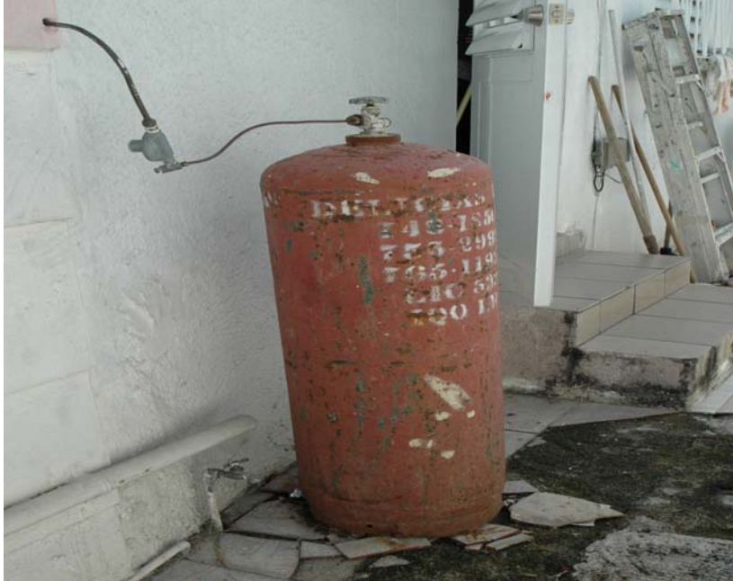
Unsecured propane gas tank outside of kitchen wall, placed over loose and broken tiles.
