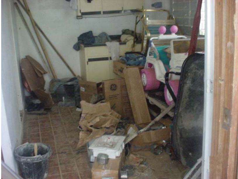
Tools, toys, and other rubbish accumulated throughout room. The tenant stated that this room is used by the owner as storage space.
