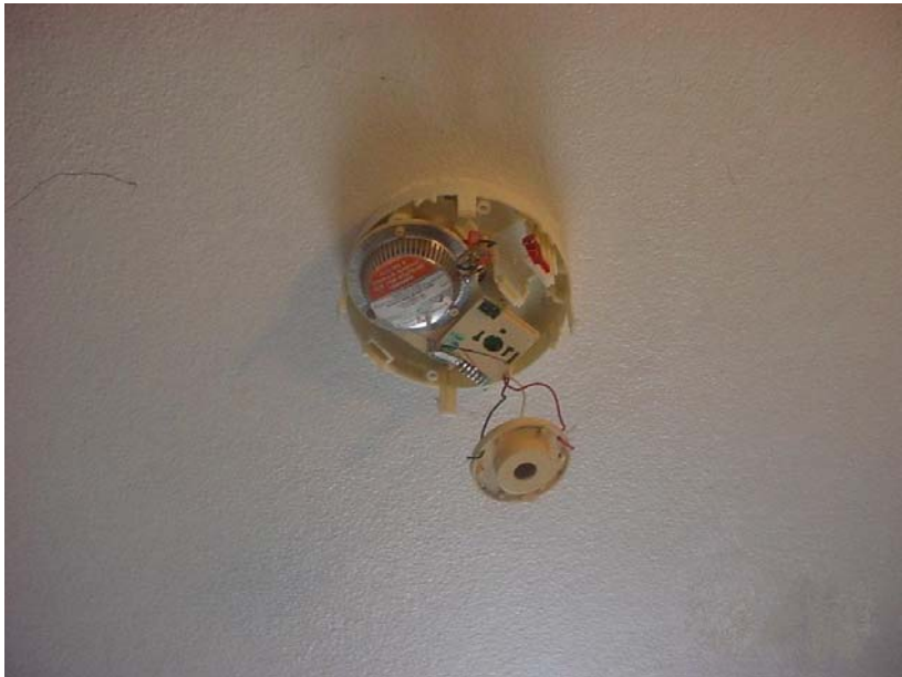
Inoperable smoke detector.
