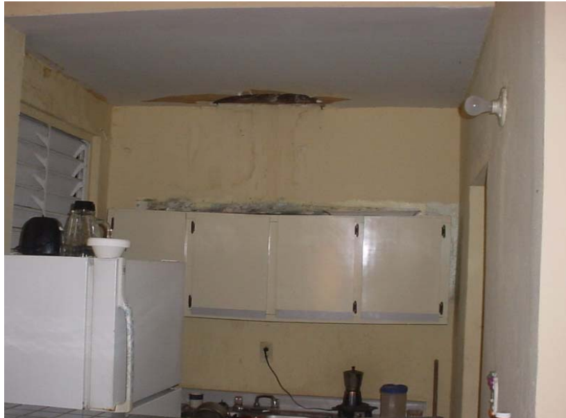
Hole in kitchen ceiling with signs of serious water leaks.
