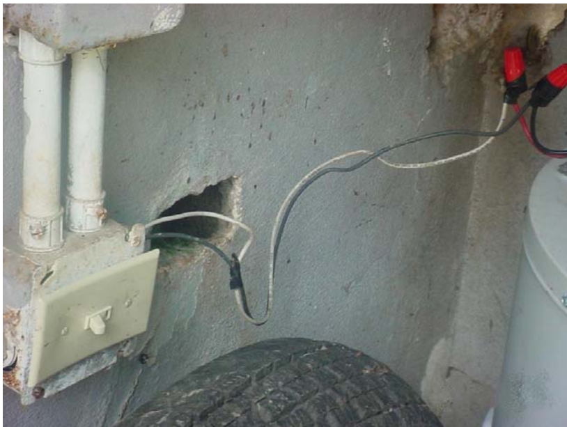
Improper wiring of water heater. The tenant stated that this deficiency existed at the time of the last Authority inspection.
