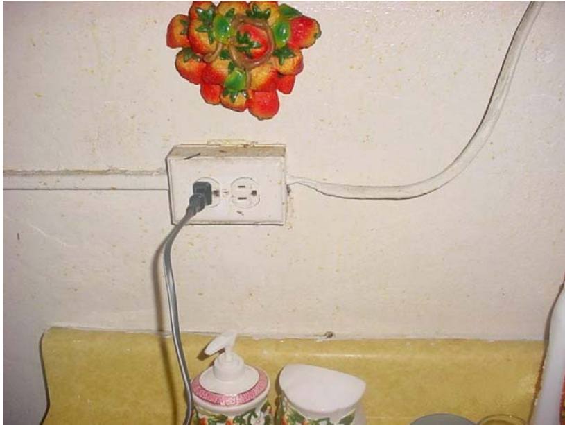
Unshielded electrical wire not reported by the Authority during its August 5, 2005, inspection.
