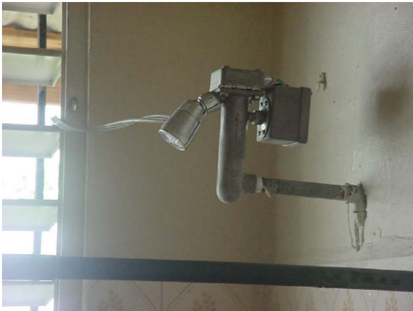
Unauthorized and improperly installed shower heater, creating an electrical shock hazard. This deficiency was not reported by the Authority during its August 5, 2005 inspection.
