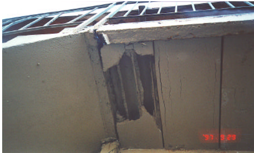
Balconies providing access to Highland Heights units showing signs of potentially dangerous structural deterioration.
