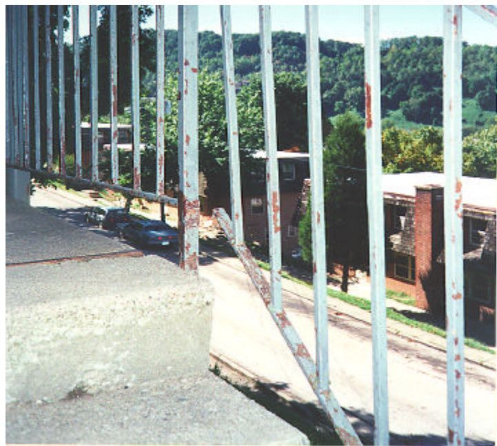
Hazardous broken balcony stair rail at 116 Highland Heights. Note height from ground.
