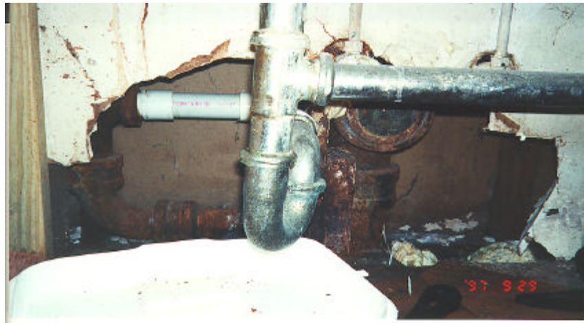
Hole in wall not repaired following plumbing repair in unit 108B Highland Heights.
