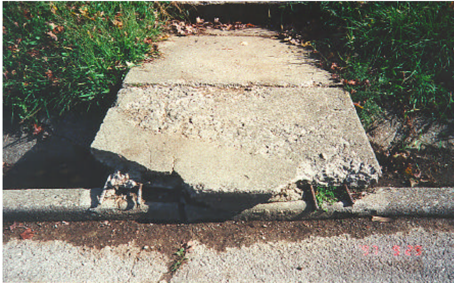
Serious walkway deterioration at Highland Heights.
