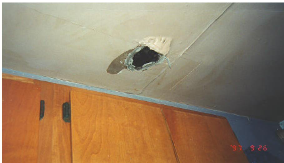
Commode leak from bathroom above kitchen in unit 156D Highland Heights.
