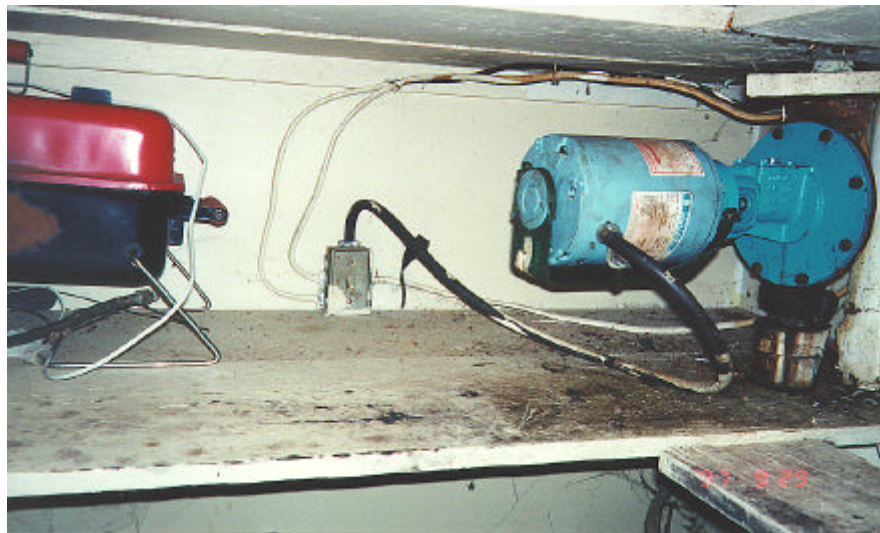
Example of unprotected wiring in Highland Heights pantries. Exposed wiring must be in conduit.
